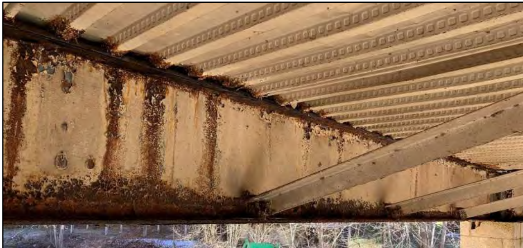
Image 16: North Landing Underside Corrosion
