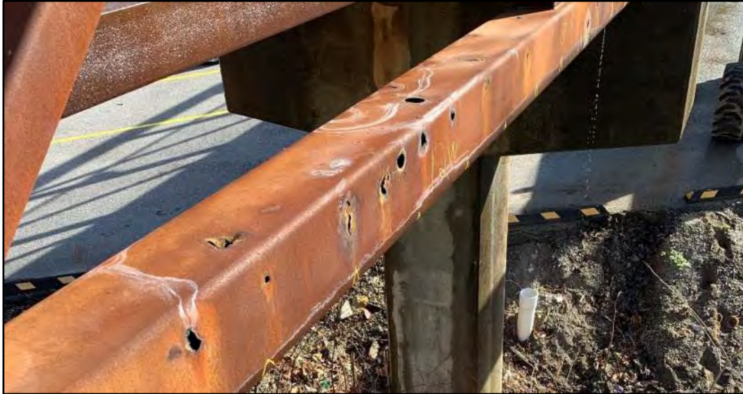
Image 6: Span 1, West Bottom Chord Deterioration
