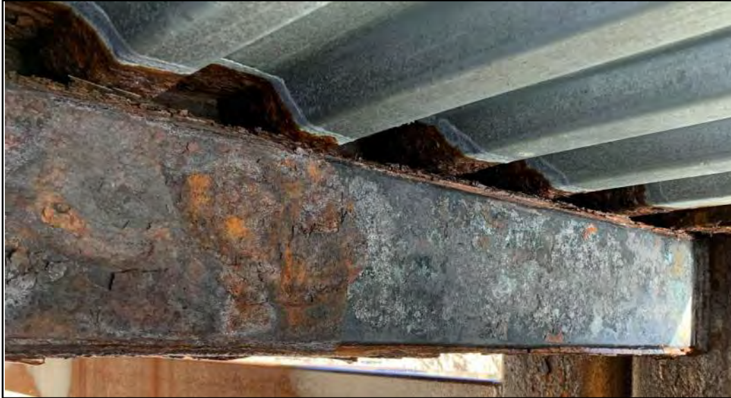
Image 2: Delamination Removed from Cross Member
