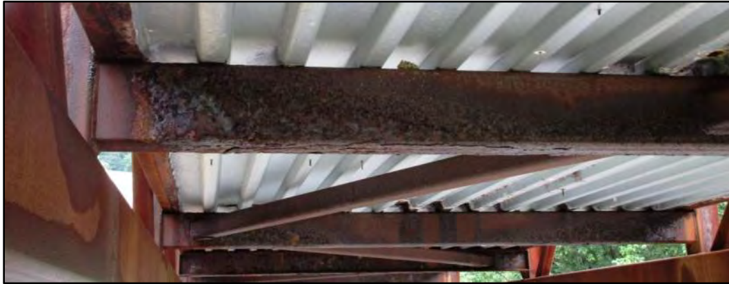
Image 9: Cross Member Corrosion
