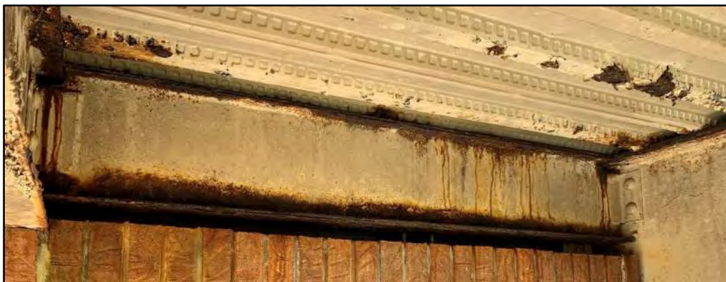
Image 17: Beam Corrosion at Building Intersection
