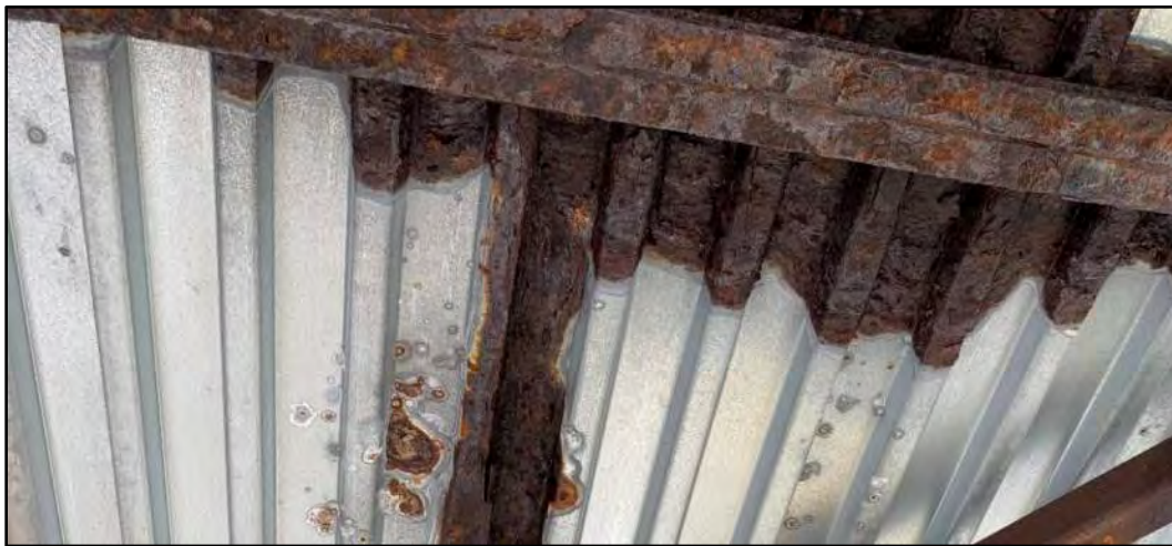
Image 11: Underside of Deck Corrosion
