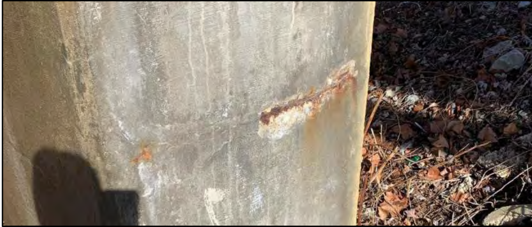
Image 13: Concrete Pier Spall
