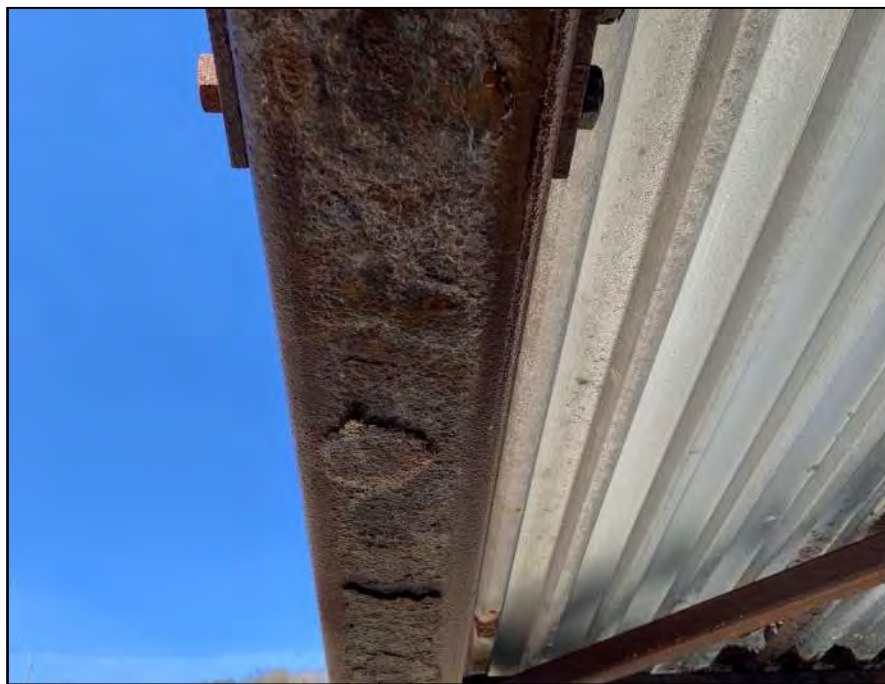
Image 8: Underside of Bottom Chord Delamination
