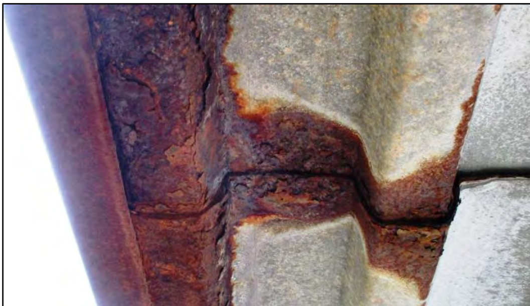
Image 12: Weathering Steel/Galvanized Deck Interaction
