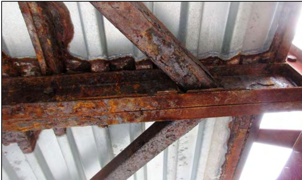
Image 10: Lateral Bracing Corrosion
