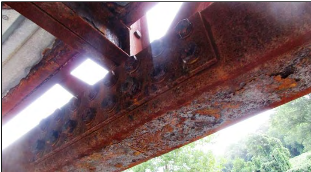
Image 14: Bottom Chord Splice Corrosion
